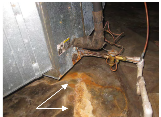
Crawl space vapor barrier is rust stained below the a/c indoor coil metal case (left side view)
