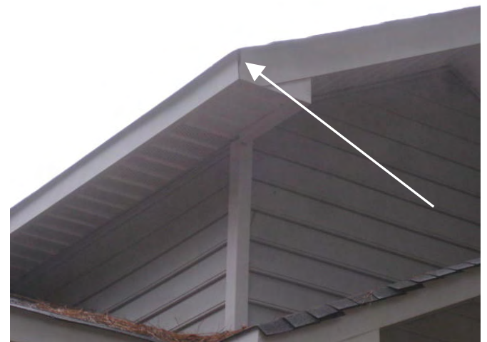
Main gable roof left side rear rake and fascia aluminum cladding vertical corner joint has a gap present
