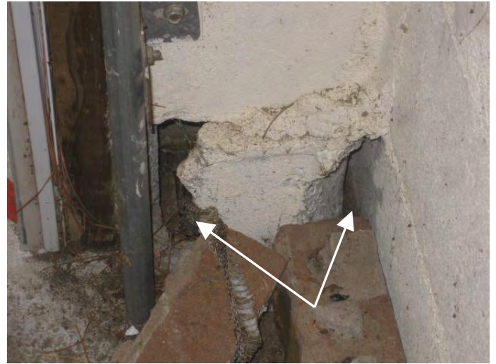
Garage right side front masonry wall lower concrete block is damaged, visible from inside the garage
