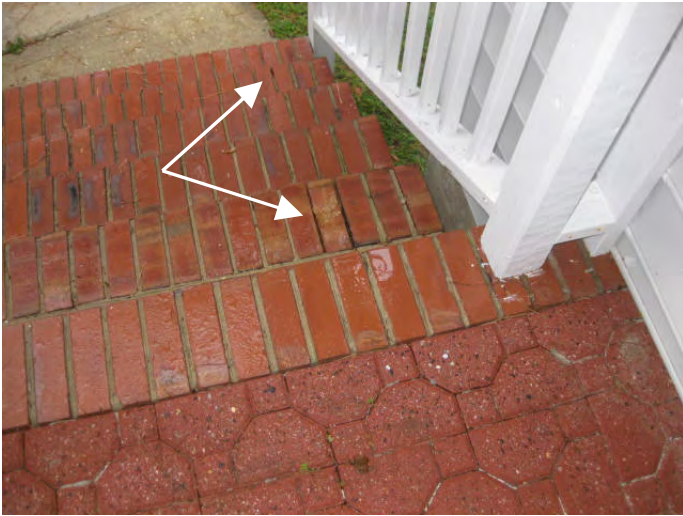
Front porch brick steps has several mortar joints with voids present
