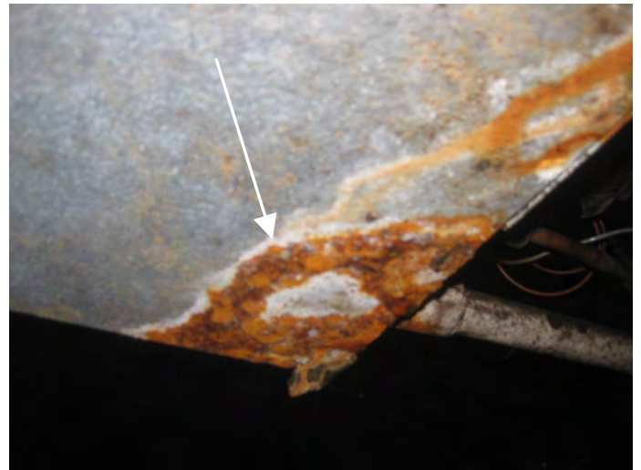
A/c indoor coil metal case is rusted (bottom view)
