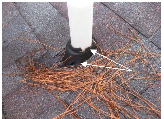
Both plumbing vent pipe roof penetration flashings (boots) are damaged, visible from the roof
