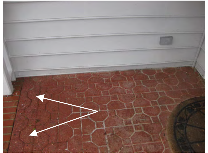
Front porch masonry pavers has several joints that are missing the mortar
