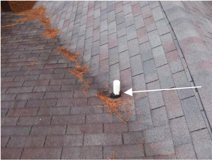
One plumbing vent pipe is currently located in a valley area
