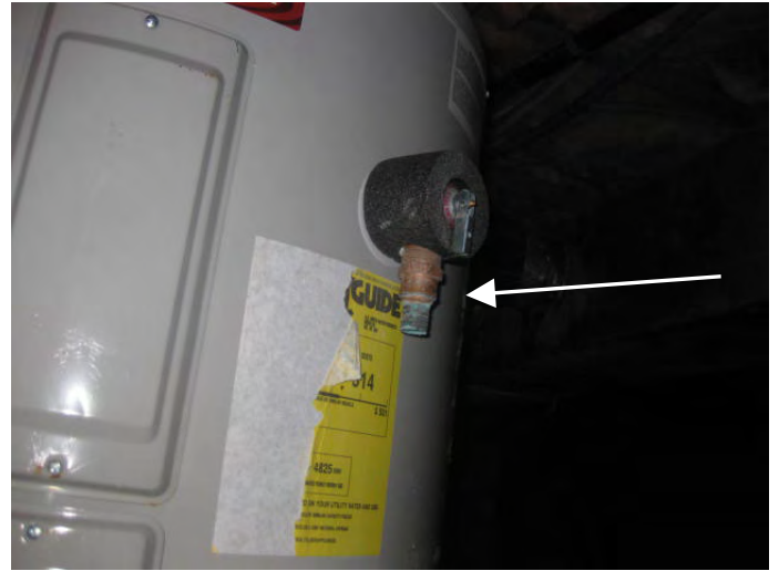
Water heater temperature and pressure relief (T&P) valve is not properly plumbed to with-in six inches of the floor (ground)
