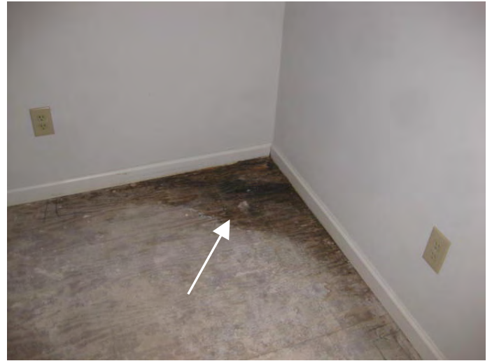
Master bedroom floor sheathing is moisture stained and tests as having a slightly moisture content in the stained area
