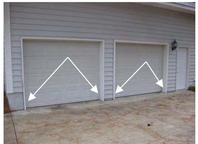
Garage right side vehicle door opening doorjamb aluminum cladding is damaged near the bottom
