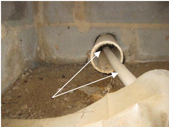
A/c primary condensate drain pipe is currently routed the foundation positive drain pipe, which looks to be clogged
