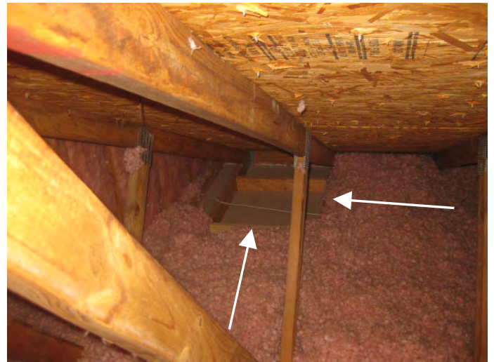
One section of the front left living room ceiling is missing the insulation along the foyer side, visible in the attic
