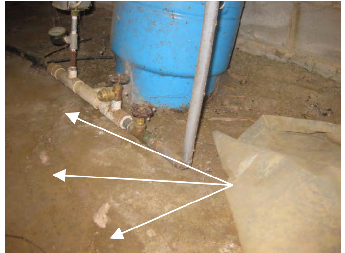
Crawl space soil and vapor barrier show evidence of surface water flow along the left side
