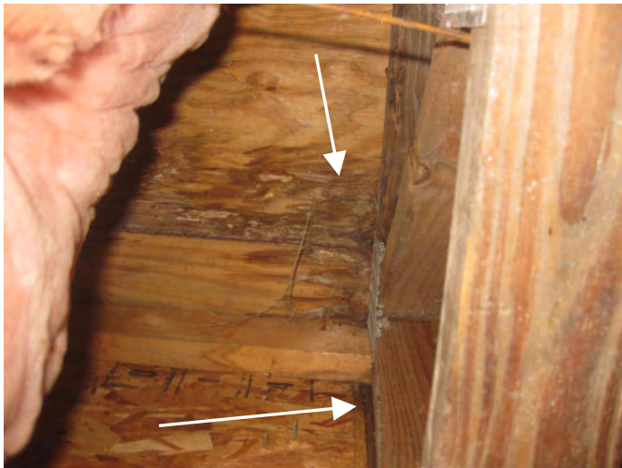
Floor framing is moisture stained below the master bathroom shower area, visible in the crawl space
