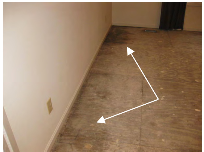
Front left living room floor sheathing is moisture stained and tests as having a slightly higher moisture content in the stained area
