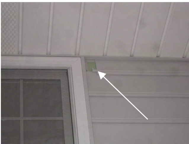
Right side upper course of vinyl siding does not completely cover the wall, located above the right side exterior water faucet area
