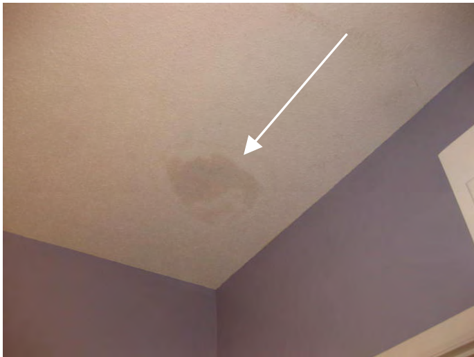
Master bathroom ceiling is moisture stained near the rear right corner (below the damaged plumbing vent pipe boot)
