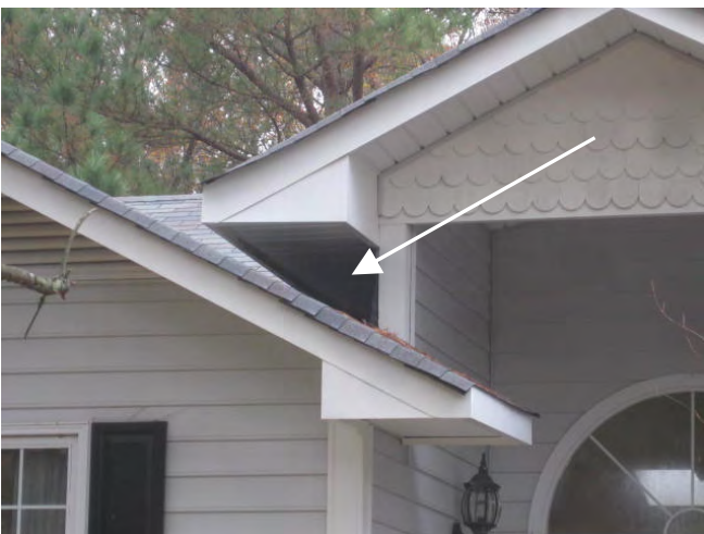
Front roof construction detail creates a high possibility of rainwater leakage
