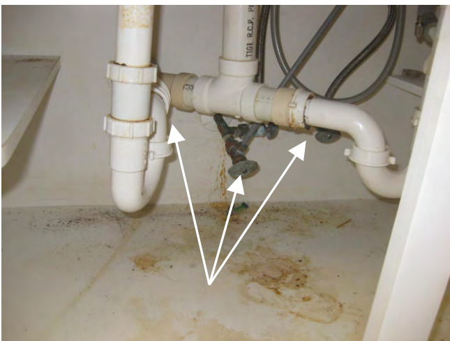
Kitchen sink drain pipes are leaking, and the water faucet hot water supply pipe shut off valve is leaking
