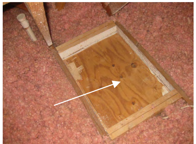
Attic scuttle hole cover panels are not properly insulated, visible in the attic (scuttle above the master commode room)
