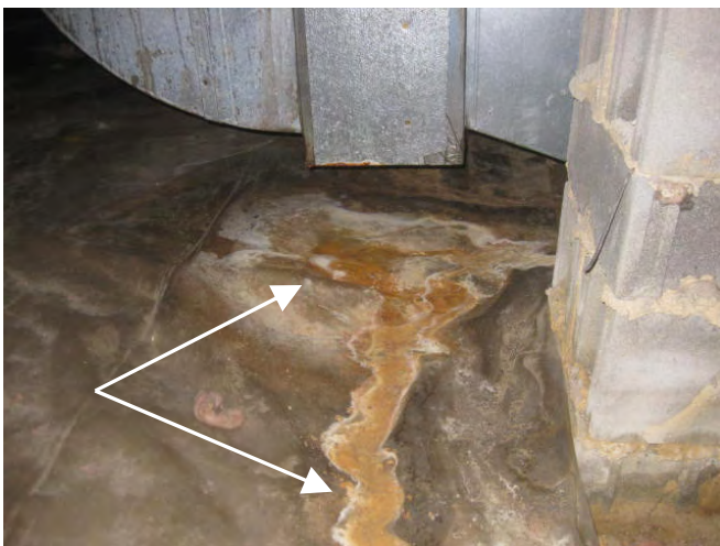
Crawl space vapor barrier is rust stained below the a/c indoor coil metal case (right side view)
