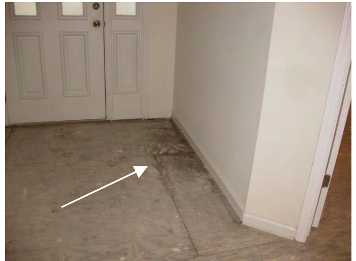
Front foyer floor sheathing is moisture stained and tests as having a slightly higher moisture content in the stained area
