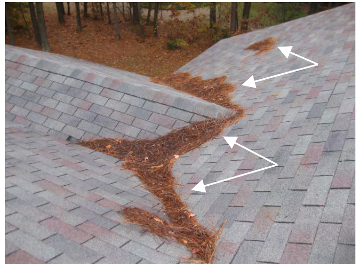
Tree debris present on roof shingles blocks visibility of shingles in some of the valley areas
