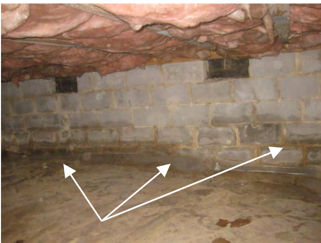
Front masonry foundation wall shows evidence of moisture penetration, located along the dining room front wall area
