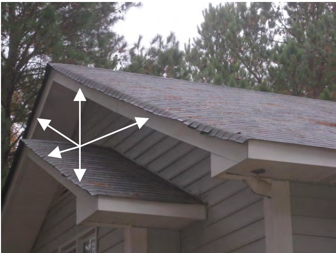
Most areas of the gable roof shingles extend too far beyond the rake edges
