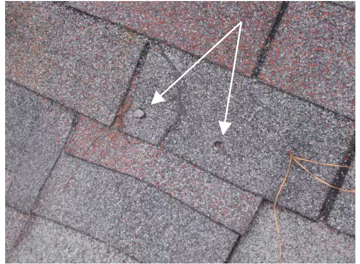
Roof ridge cap termination shingles face nail heads are missing the roof sealant
