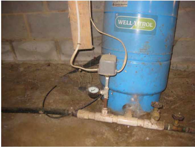
Well pump short cycles during water use
